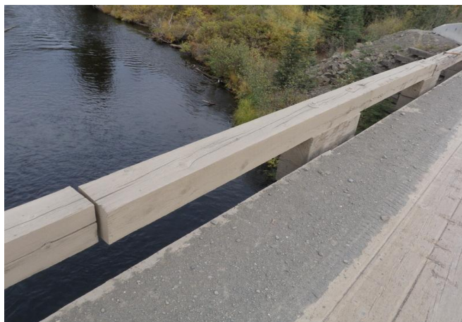
Figure 1-14: Middle bridge curb rail with one unsupported end; typical on both curbs.
