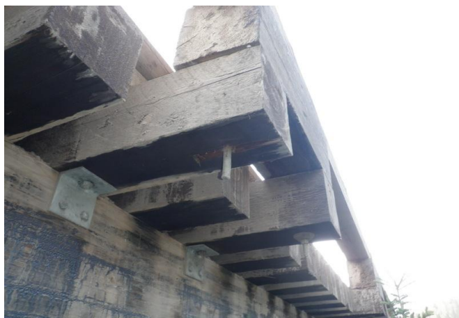
Figure 1-15: Downstream curb anchor near camp end missing nut and washer.
