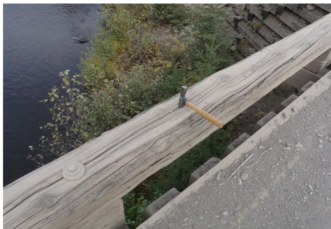
Figure 1-13: Typical longitudinal checks on bridge curb; downstream curb shown.
