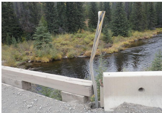
Figure 1-7: Damaged camp end downstream delineator.
