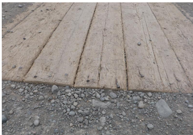
Figure 1-10: Typical end of deck condition.
