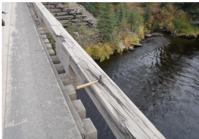
Figure 1-12: Typical pockets of rot on bridge curb; upstream curb shown.
