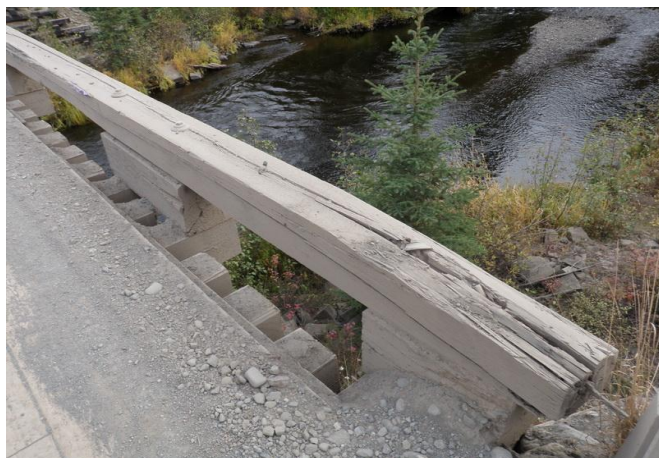
Figure 1-11: Woods end upstream curb damaged.
